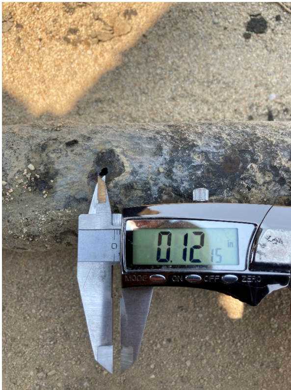
Photo 2: Hole in now-repaired pipeline.
